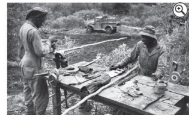
Soldiers at a makeshift bench work on the Alaska Highway in the northern sector of Alaska in 1942. The contribution of segregated Black soldiers was largely ignored for decades. In 2005, Congress passed a resolution honoring Black engineers for their efforts in the face of "indignities and double standards."
